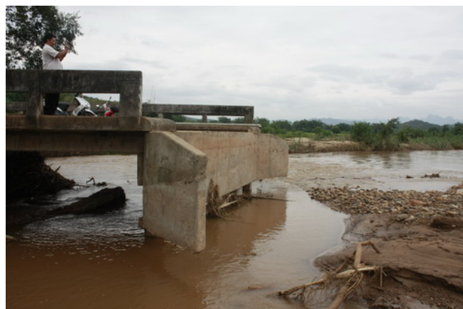
The damaged road leading to Suk jai children Home
